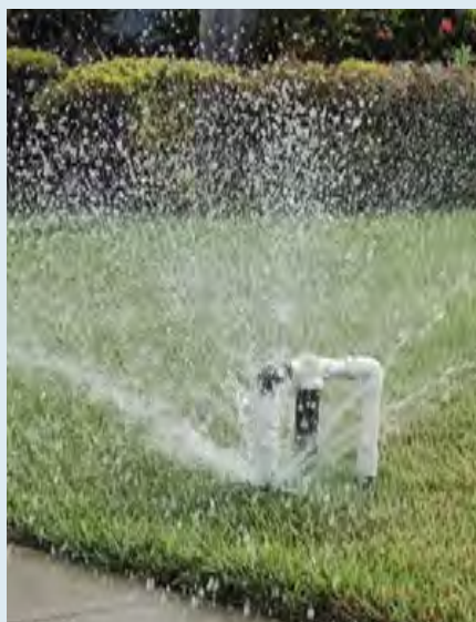
A pipe constantly under pressure sprung a leak, draining thousands of gallons before being shut off.
