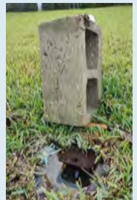
A concrete block was used to divert the spray and find the underground valve.
